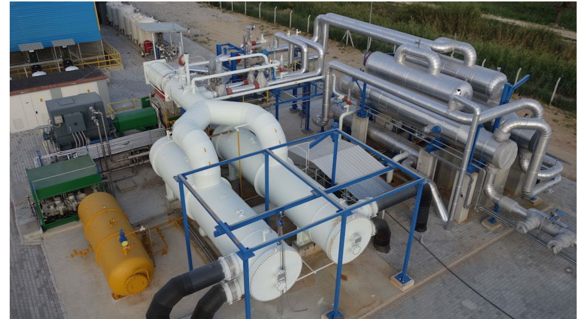
Figure 18: Example of 4MW binary plant from Denizli Tosunlar ORC geothermal power plant, Turkey [20] [21].
